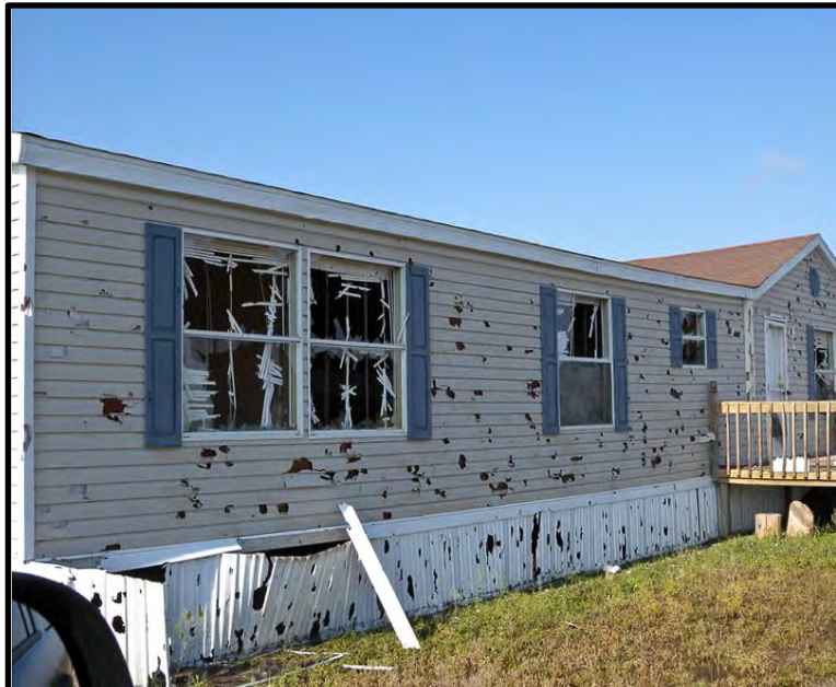
Significant mobile home damage from hail. Source: NSSL
